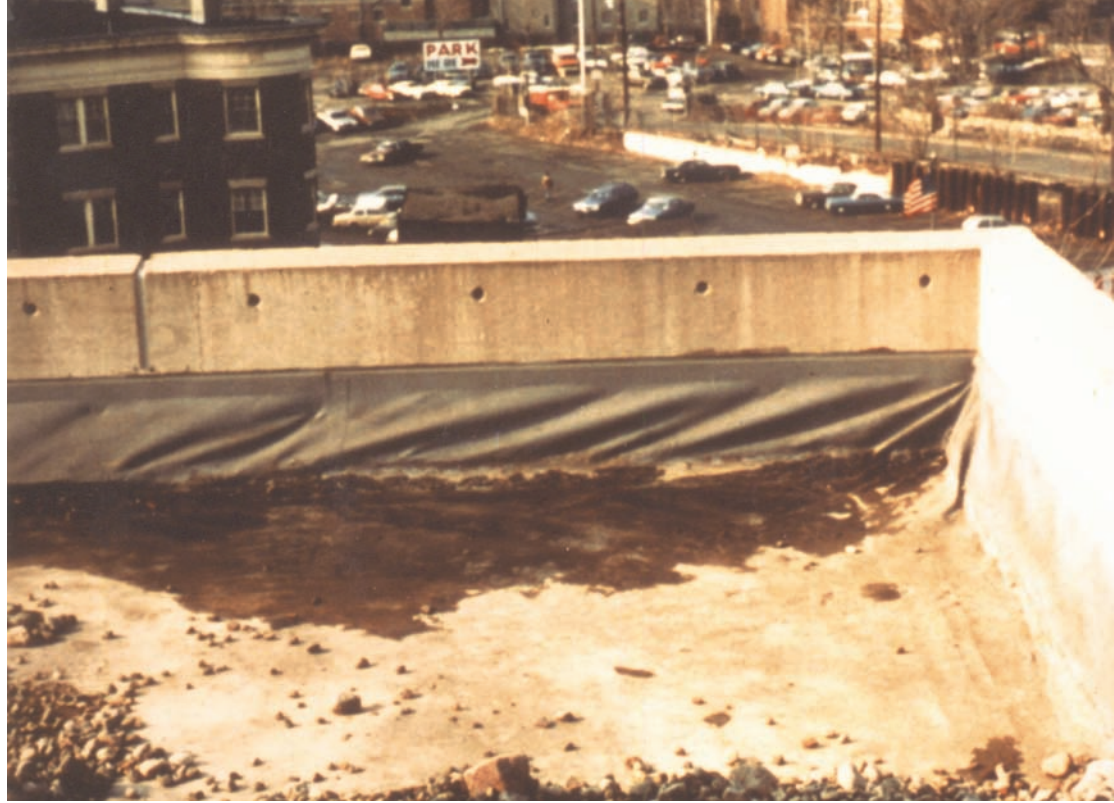
Figure 2—Differential building movement which ruptures a membrane is a legitimate warranty disclaimer. Water will likely enter the building with no help from the long-duration roof warranty.
