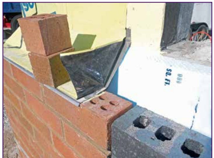
Figure 4 – Full-scale mock-up of a TWF condition on a new construction project. The design intent includes full support for the self-adhering membrane through the wall cavity.
