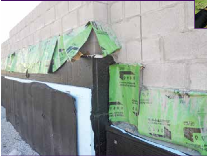
Figure 2 – Sight to be “unseen”—the birthplace of future performance issues with a through-wall flashing (TWF) condition.
