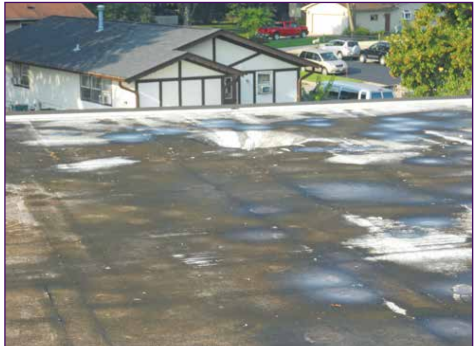
Figure 9 – The roof in this figure was designed by a manufacturer, with the owner under the impression that the service constituted “added value.” No efforts were made to improve drainage. Minimally, a tapered insulation section or sump at the drain heads would have been added value.
