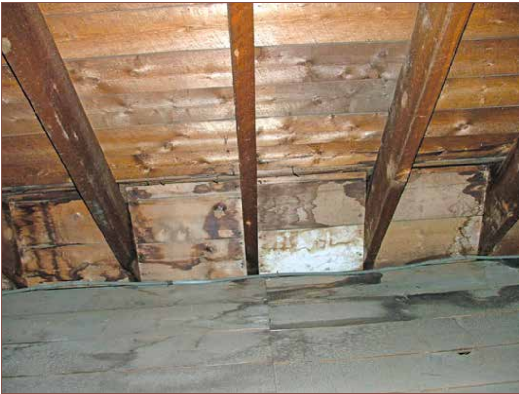
Figure 4 – Staining under roof deck and on floor.
