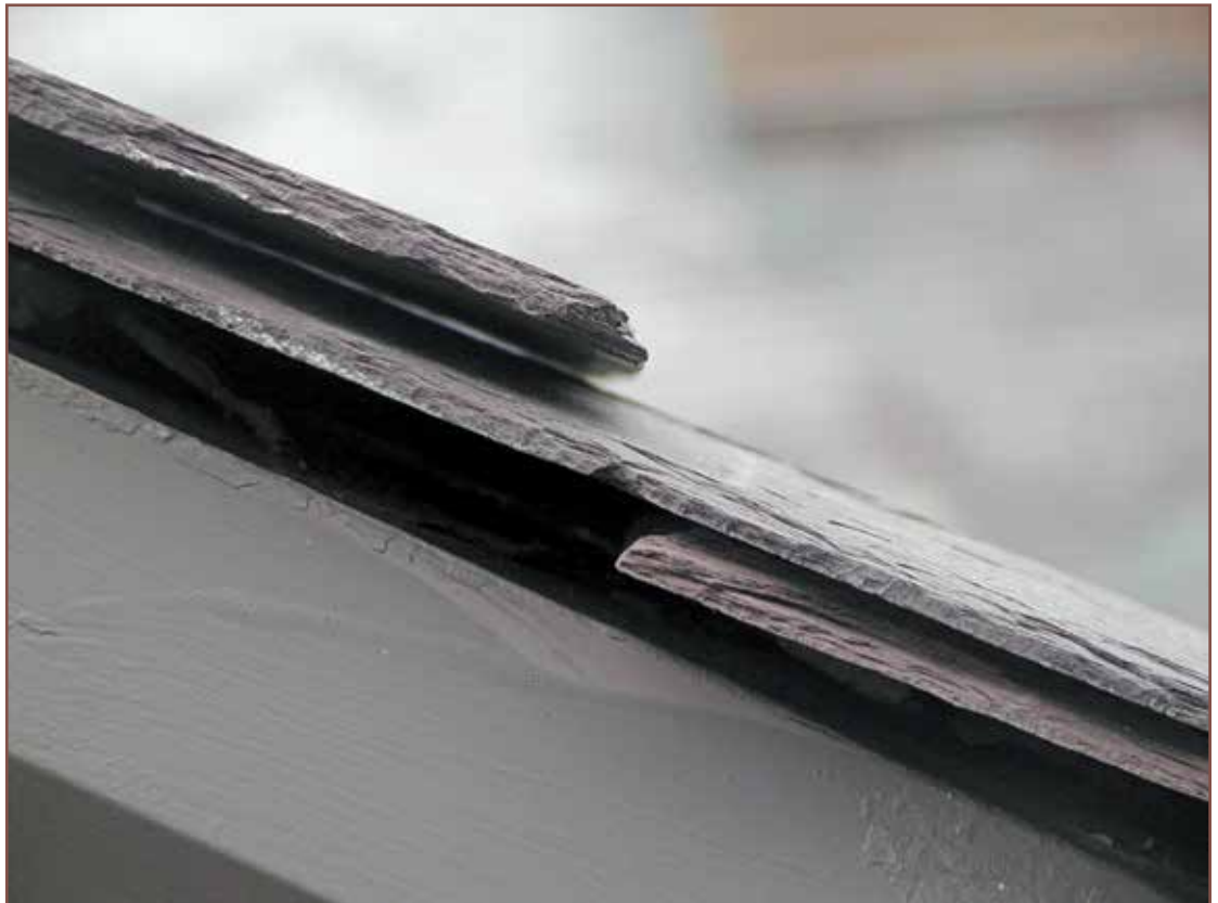
Figure 3 – Improper head laps.
