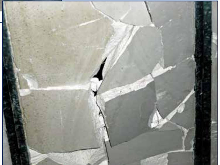
Figure 9 – Without embedded wire reinforcing, this compromised deck would surely have fallen. Note the “white” core, indicating that this is a gypsum product.
