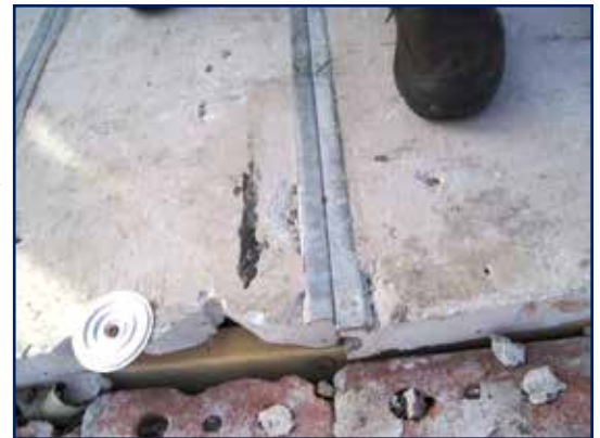
Figure 7 – Just as with openings in other deck types, these panels need support bracing where the continuity of tongue-and-groove edges is violated. This can be as simple as anchoring a lumber ledge band or adding red-iron framing members. The issue is to determine how panels are terminated and how any unbraced fractions are addressed. (Image courtesy of Scott Hinesley.)
