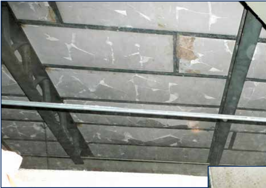
Figure 8 – Example of damage needlessly inflicted on precast lightweight cementitious planks. Contractors working on such a deck should diligently research the proper type and size of fasteners.
