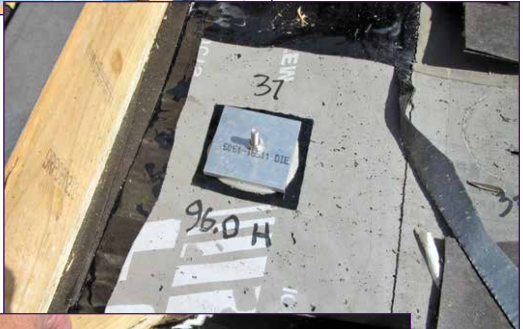
Photo 6 – At test location #37, using 2-in.-square loading fixture, 96.0 pounds of vertical (tensile) force was not sufficient to pull the flashing plug from the stucco.
