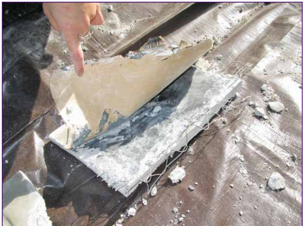
Photo 1 – Delamination of layered flashing product due to strong bonding of base membrane and stucco.
