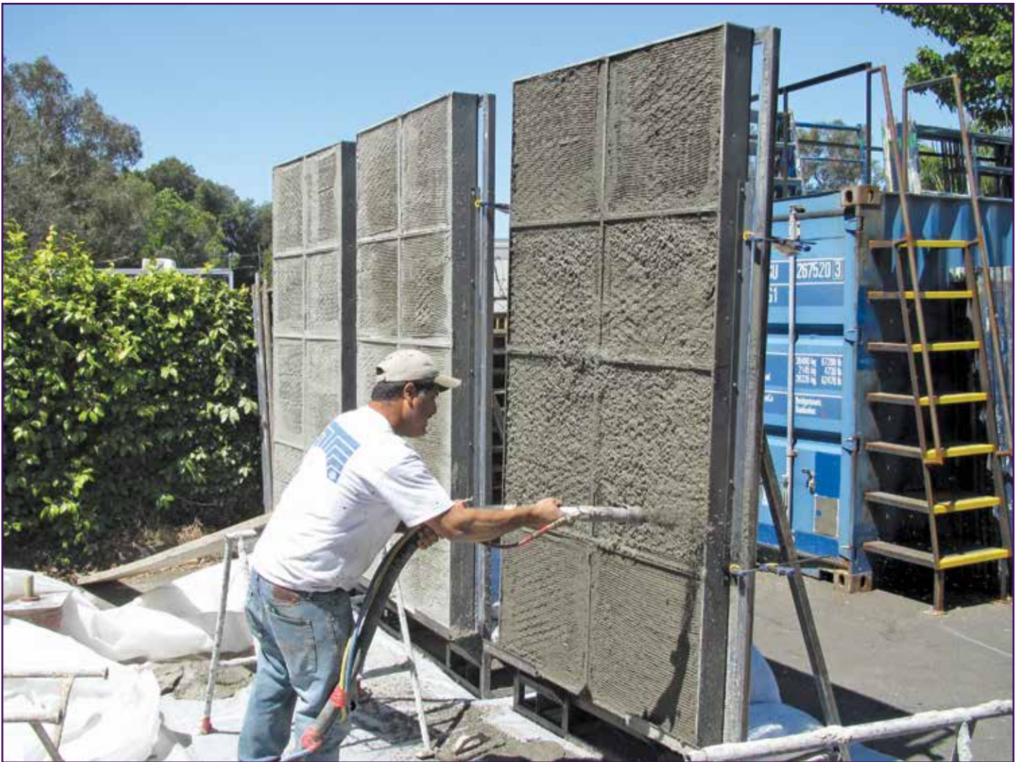
Photo 8 – Typical pump (or “gun”) application of stucco brown coat atop prior scratch coat.
