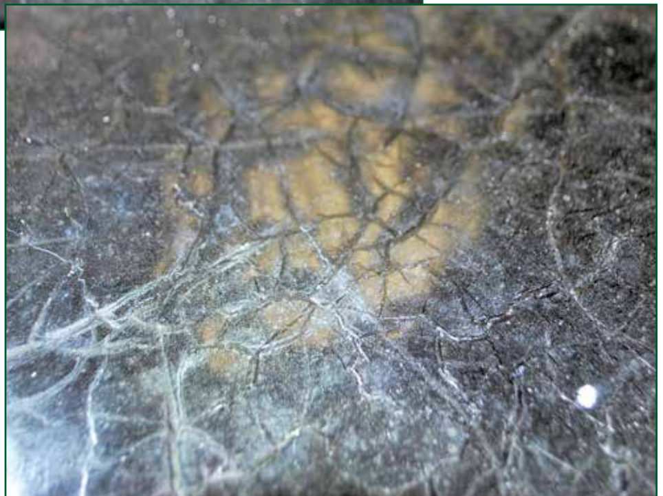
Figure 2 – Surface of SBS-modified bitumen that has been exposed to unfiltered ultraviolet radiation for 1,500 hours.
