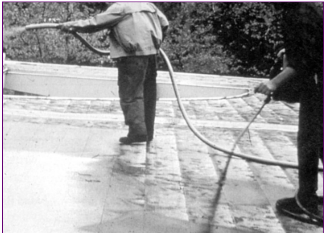
Fig. 1: A cold-applied system is being finished. One workman is spraying adhesive while another blows in granules to give a smooth, reflective surface. Courtesy: Contractors Guide, August 1990.
