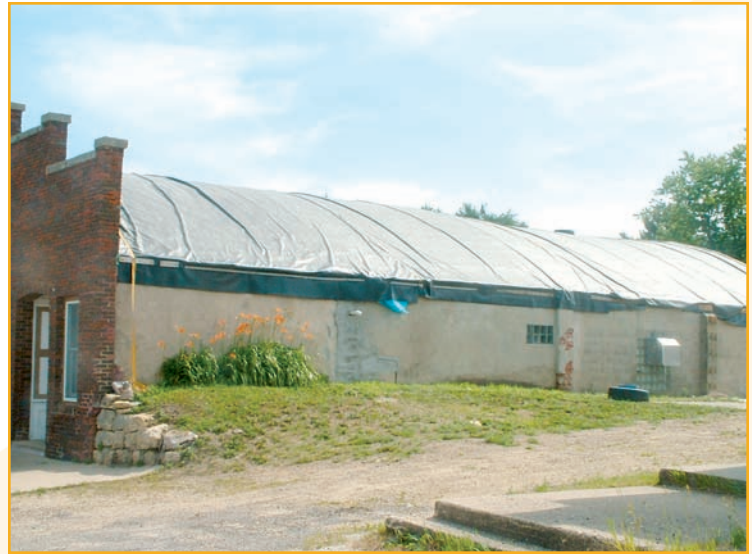
Photo 5. The ratchet straps on the barrel ends holding down the roofing are not clearly visible. Although an extreme case, the materials that are visible are FM- and UL-approved. Specification of approved materials is not necessarily a good assurance of performance.
