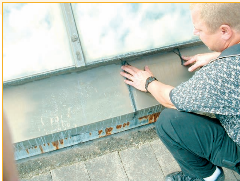
Photo 3. Roof consultants are extensively involved during the pre-design and design phases of a project. Here, an owner's representative is inspecting existing flashing details with a roof consultant.
